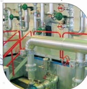
<< Industrial Process Systems
